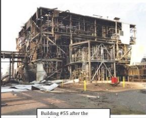
Building #55 after the explosion
