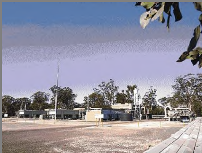
Section of gas extraction plant infrastructure at present operating at AGLs Rosalind Park site
